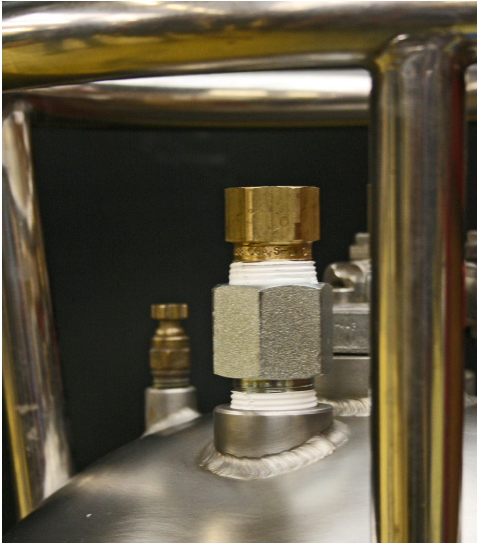
Figure 4. PRV Adaptor & PRV installed.
